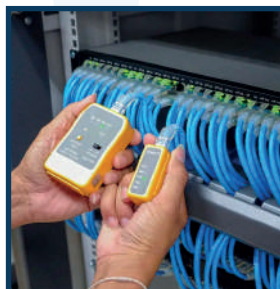
Network & Structured Cabling Solution
